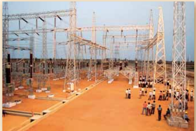
220/33KV Vajrakarur Substation, Anantapur, A.P.
